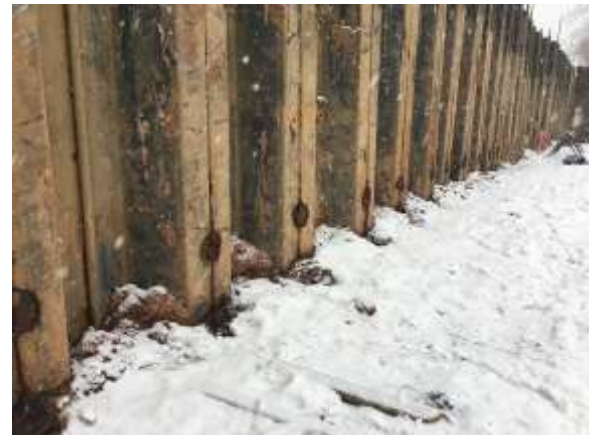
Removed pieces of the sheet piling in preparation for the tiebacks to be installed.
