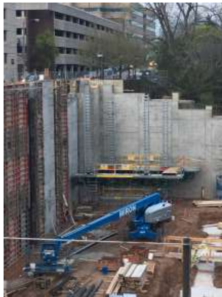
The platform pictured above is a lift used by the masons when erecting the elevator shafts.
