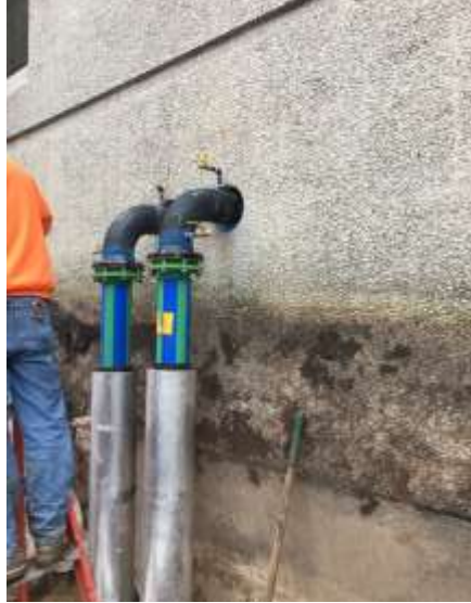
The new chiller lines being installed through the north wall of the Radisson Paper Valley Hotel.
