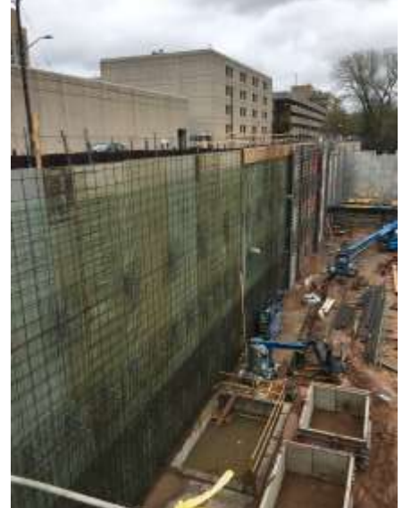
Extent of the rebar work in the north wall along Lawrence Street.
