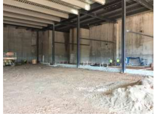
Masons started the interior CMU walls within the exhibition center. Plumbing rough-ins are also taking place.
