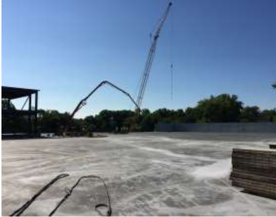
There were three major concrete pours this week; the final pour took place on 7/7. The first layer of the plaza level roofing system is now complete.
