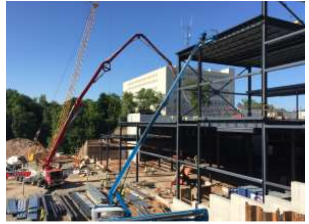
On 7/7, the last concrete pour was made at the plaza level. Steel workers are finalizing the placement of steel decking.
