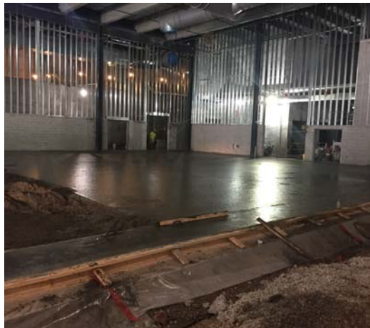
The south third of the expo hall floor was poured and completed on 9/22. The next concrete floor pour will be the north third of the expo hall.
