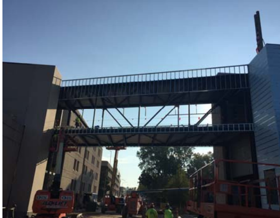
Masons have started on the interior stone. The crosswalk slab is poured, and exterior framing has begun.
